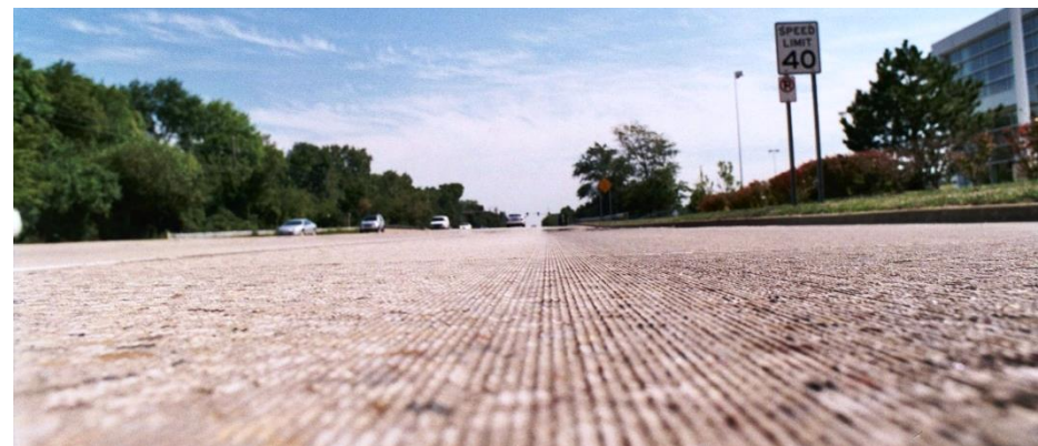
Figure 34: Pavement After Diamond Grinding (John Roberts). This picture shows the texture of PCC pavement after diamond grinding was used on it. The image was taken on a project near Chicago Illinois.
