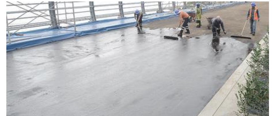
Figure 30: Slurry Seal Being Placed by Hand (Miraflores) This slurry seal is being placed to refresh the surface of the Villeno Rey Bridge in Miraflores, Peru.
