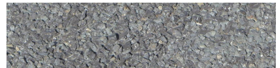
Figure 32: Close-up View of Chip Seal Surface This close-up picture of a road that has been chip sealed shows how coarse the application is and how aggregates tend to be looser on top of the new surface compared to other treatments that evenly mix the aggregate into the binder.
