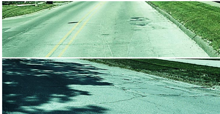
Figure 20: Example of "Very Poor" Condition (HMA) – Greene Street This image shows an HMA street whose pavement is rated as 20/100 and considered to be in "Very Poor" condition. Greene St west of 11 th is considered the worst HMA surface street in Adel due to deep ruts and large localized failures.
