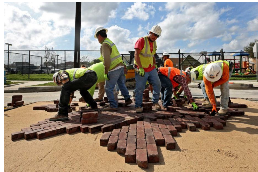
Figure 39: Crew Manually Re-laying bricks (Godofredo A. Vasquez) This crew in Houston is laying historic bricks in Freedmen's Town.
