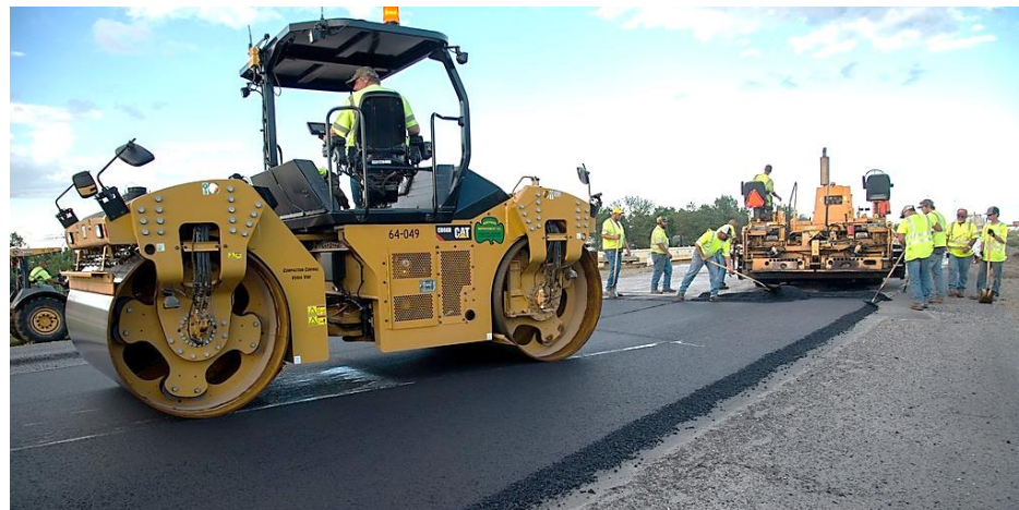
Figure 26: Reconstruction of I-94 (NDDOT) This photo shows the Construction of a brand-new asphalt cement concrete pavement
