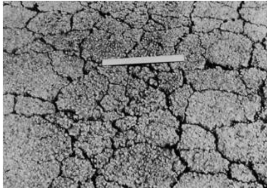
Figure 5: Example of Alligator Cracking (ASTM)
