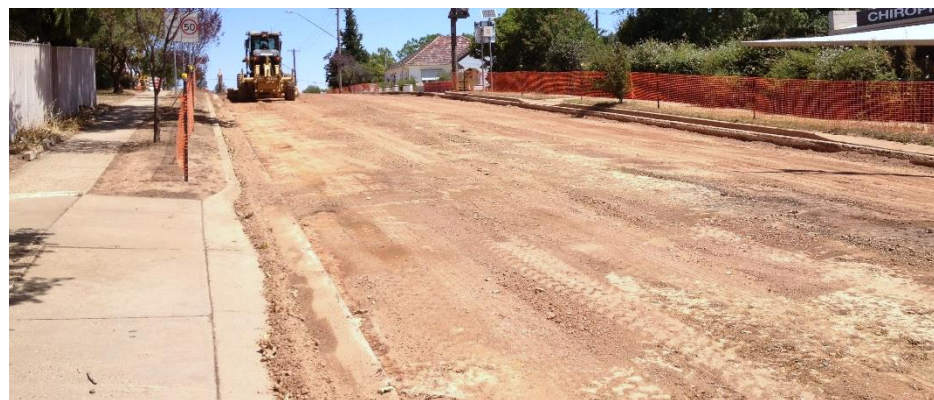
Figure 27: Reconstruction of Michelmore Street (Bidgee) This photo shows a road torn out and being prepared for reconstruction
