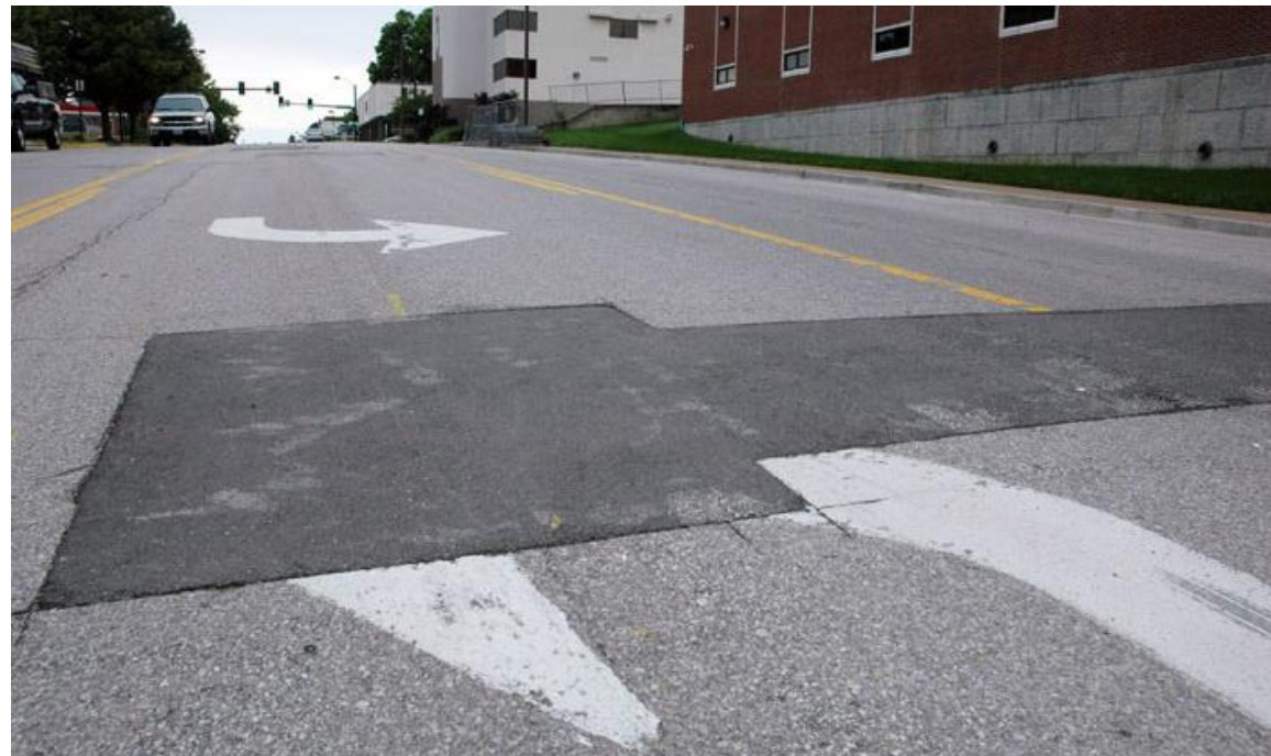
Figure 37: HMA Patching with Localized Pavement Removal (KOMU) This is an example of an asphalt patch applied with appropriate localized removals and some base repair.
