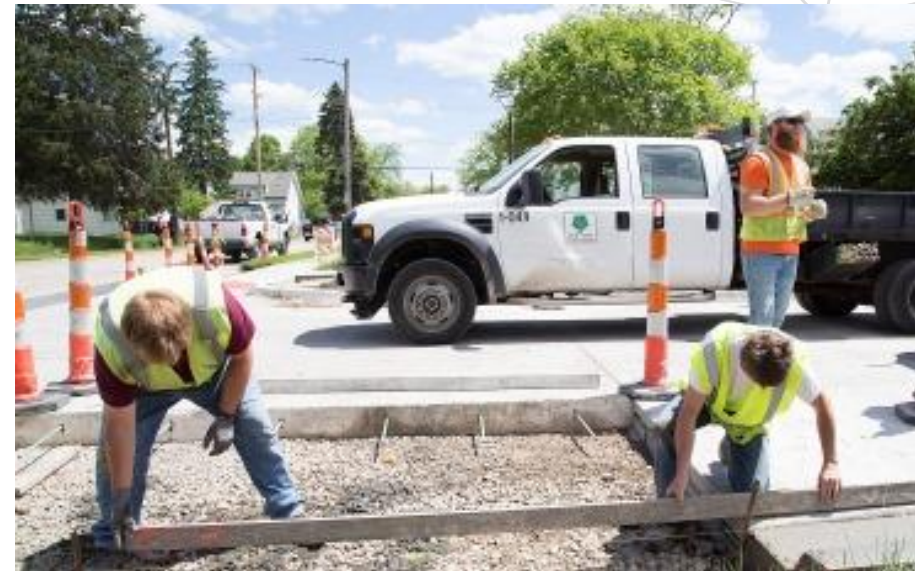
Figure 33: PCC Restoration (City of Cedar Rapids). This is a picture of a city maintenance crew in Cedar Rapids performing a panel replacement as part of a larger concrete restoration project.
