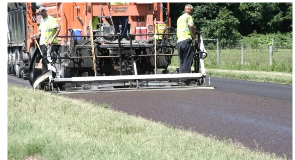
Figure 31: Microsurfacing Crew at Work. (Eric Pulley). This picture shows a crew using a Microsurfacing machine to lay a new surface on this street.
