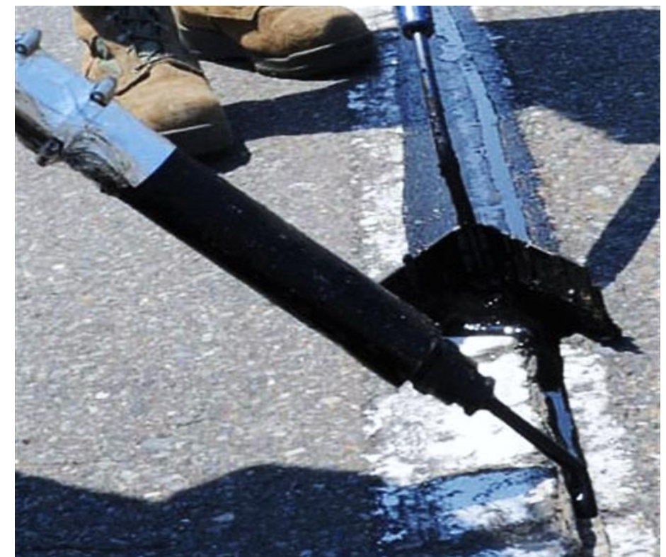
Figure 36: Crack Sealing Performed W/ Routing (USAF/Kenna Jackson) This is an example of crack sealing being performed with special preparation in the form of using a router to clean up the crack profile, as being performed by 35th Civil Engineer Squadron.
