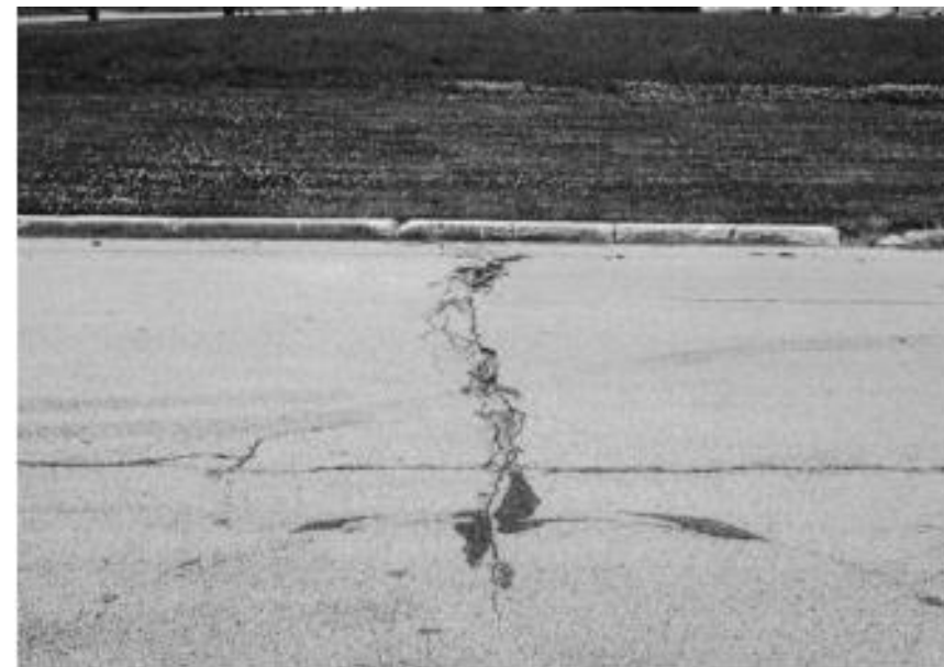
Figure 8: Example of Transverse Crack (ASTM)
