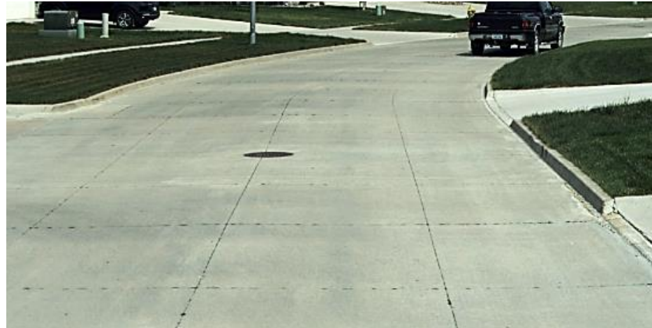
Figure 13: Example of “Very Good” Condition (PCC) – Shelby Drive This image from the 2021 data collection shows Shelby Dr near Meadow. It was rated as a-perfect 100/100 and would be considered “Very Good” for a PCC pavement.
