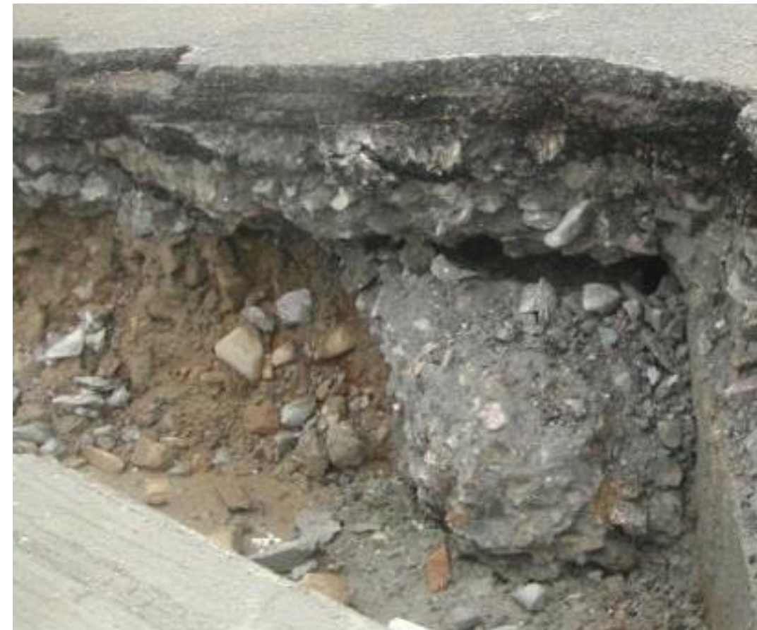
Figure 61: Under Pavement Voiding (Chen) This photo shows a pavement void that has formed along the bottom of a pavement due to subgrade issues.
