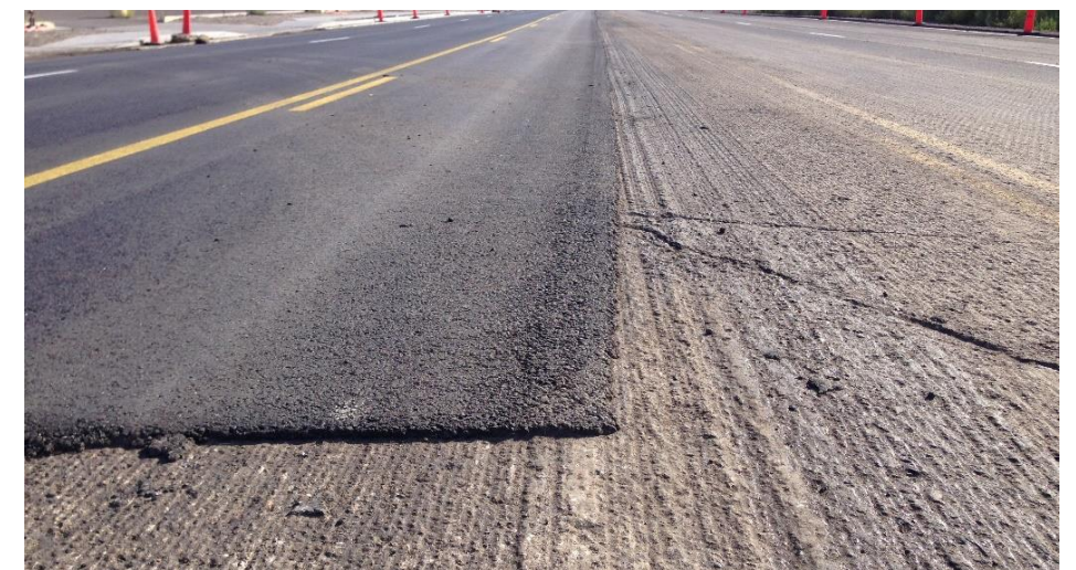
Figure 28: HMA Overlay Placed On Milled Pavement (Famartin) This is a picture of an asphalt overlay placed on I-80 through Elko, Nevada after part of the original pavement was milled off.
