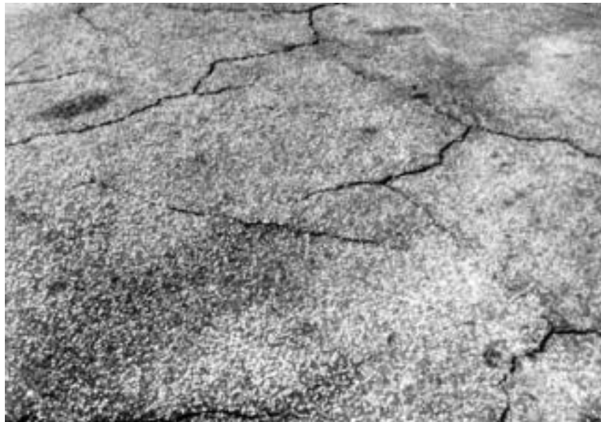
Figure 6: Example of Block Cracking (ASTM)
