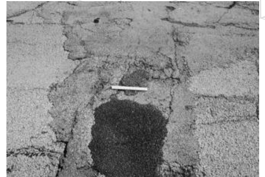
Figure 9: Example of Patching (ASTM)
