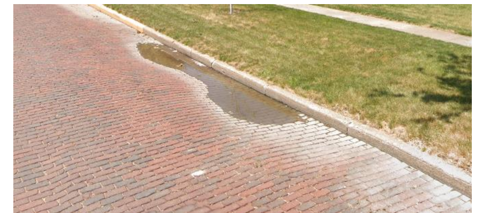
Figure 40: Area Distortion of Rapids Street Holding Water This area has distorted enough to catch and hold water, which indicates it will likely continue to fail as water and frost undermine the subsurface support.
