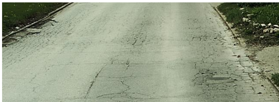
Figure 18: Example of "Poor" Condition (HMA) – Grove Street This image shows an HMA street whose pavement is rated as 30/100 and considered to be in "Poor" condition. Grove Street east of 15th has significant alligator cracking and distortions along the wheel path and pavement edge affecting the ride.
