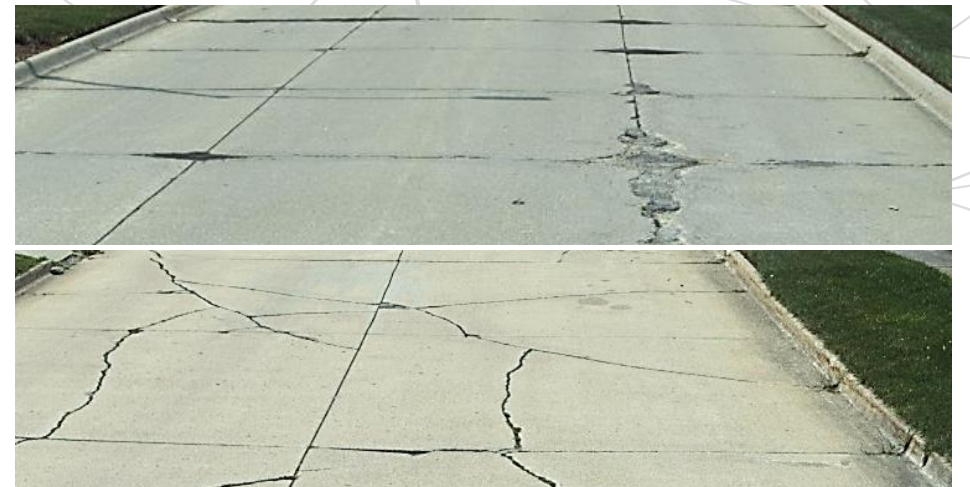
Figure 22: Example of "Very Poor" Condition (PCC) – South 16 th Street This image is an example of a PCC pavement in "Very Poor" condition. South 16 th St south of Hyvvue is considered the worst condition road in the system due to widespread joint spalling, d-cracking, most panels are cracked..
