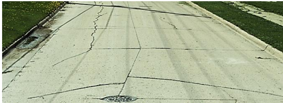
Figure 17: Example of "Fair" Condition (PCC) – Prairie Street This picture of western Prairie St is an example of a PCC pavement that was rated as 52/100 which would be considered "Fair." It has visible distress, but they are sealed or patched.
