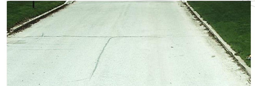
Figure 14: Example of “Good” Condition (HMA) – North 15 th Street This picture of N 15 th St north of Main was rated as 68/100, which would be considered Good for an HMA pavement. Small distortions, and a few non-wheel path cracks can be found, but nothing that impacts drivers like cracks in the wheel-path or patches of failure.
